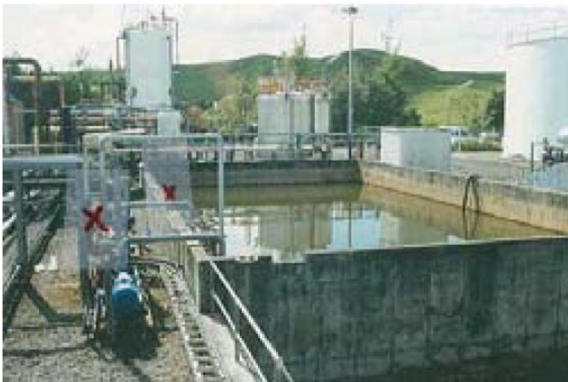
Photo 2 Treated stormwater ‘swimming pool’ STW002007
